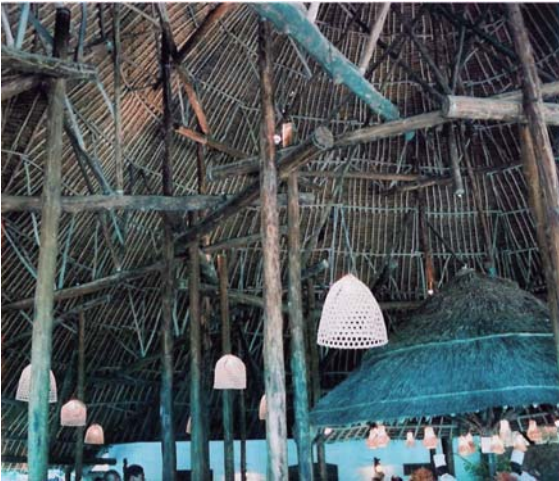
Building Construction. Fig. 11 Roof structure with tree-type supports (Beach Resort in Kenya) (photo by the author).
